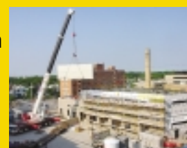
Crane places 33,000 pound generator on the roof of the new loading dock.
