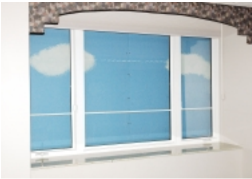
It was nothing but blue skies and fluffy clouds in Administration and part of Patient Registration as windows were boarded in preparation of removing the West Annex.
