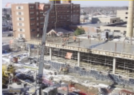
Northeast view of loading dock; concrete cement being pumped on the south end of the building.
