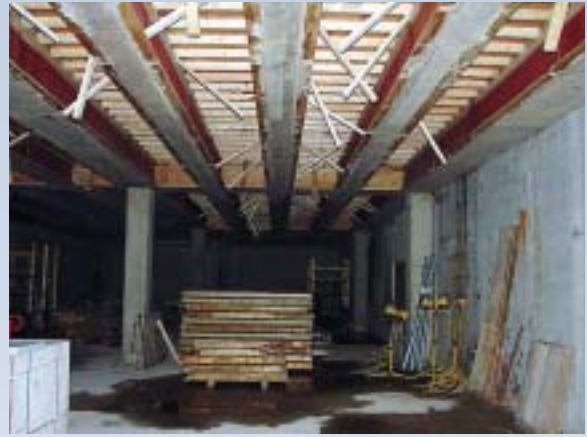
First floor of the loading dock; deck form work being dismantled off of second floor concrete deck.
