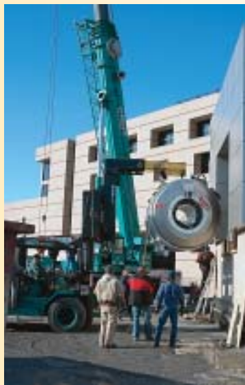
A crane was used to lift the 13-ton 3T MRI out of its temporary location and relocate it to its permanent home in the South Expansion.
